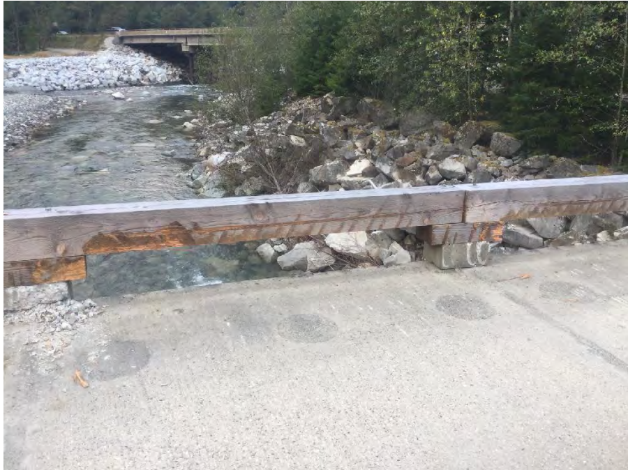
Photo 29 Curb mechanical damage
