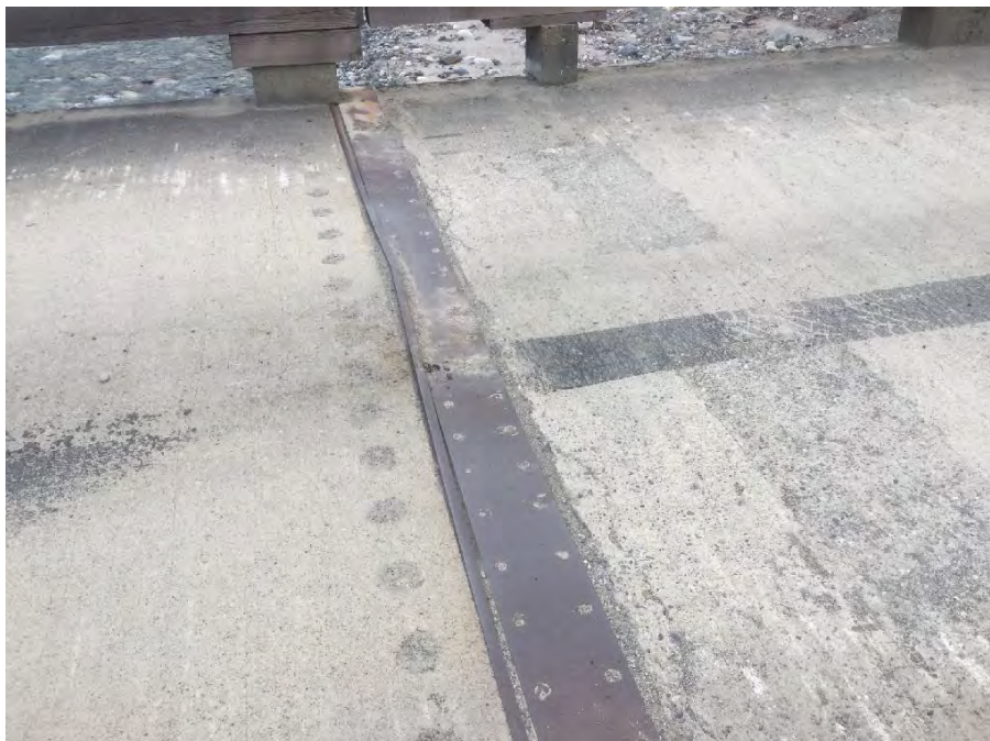
Photo 30 Expansion joint damage over pier 2
