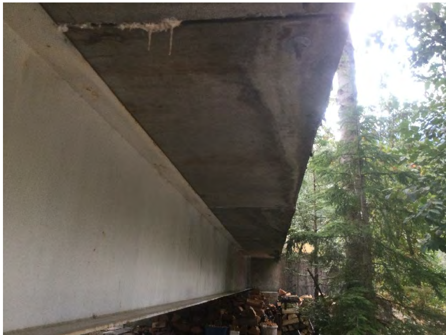
Photo 34 Exterior soffit condition showing efflorescence
