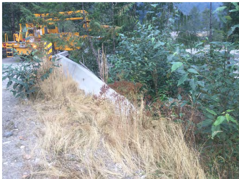
Photo 32 Left upstream barrier falling down embankment
