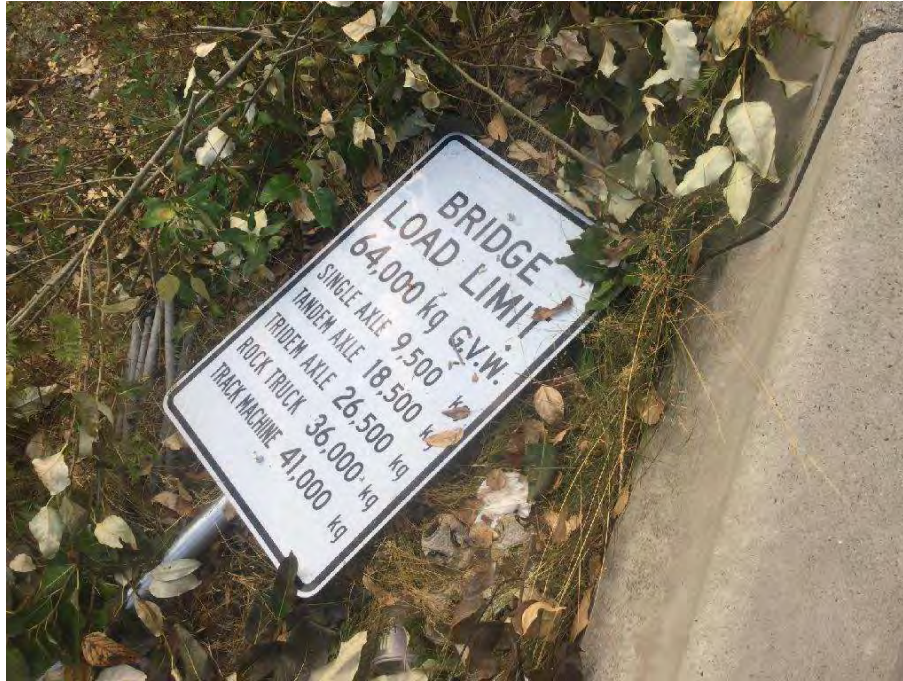
Photo 27 Right load rating signage knocked over
