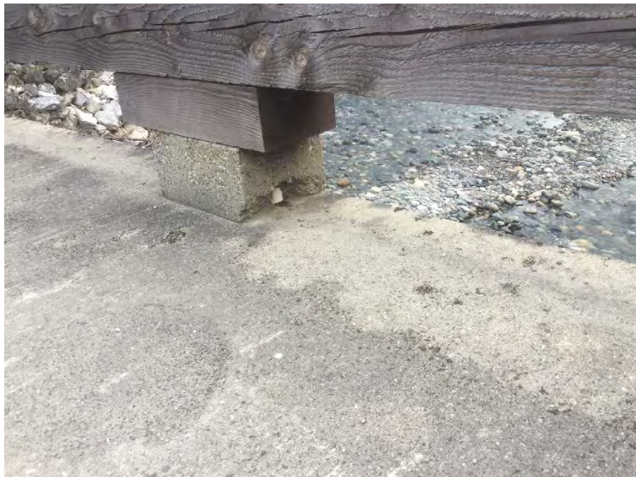
Photo 28 Concrete curb riser spalling
